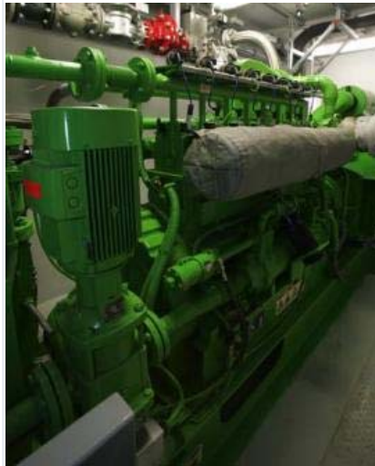
A large engine-driven generator at the KBCSI green energy project is designed to produce electricity from biogas. (Ken Love/Akron Beacon Journal)
